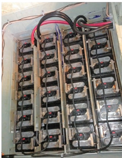
Four HuP SolarOne flooded lead-acid batteries supply 950 Ah at 48 VDC—enough storage for the whole neighborhood.
